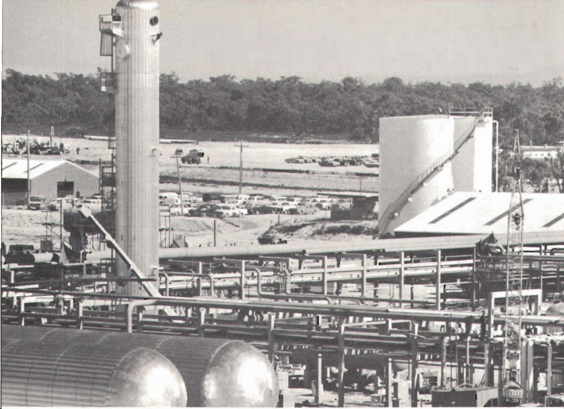
Part of the Esso—B.H.P. Gippsland plant at Dutson, near Sale, where crude oil is stabilised and natural gas is processed before being piped to Melbourne.
