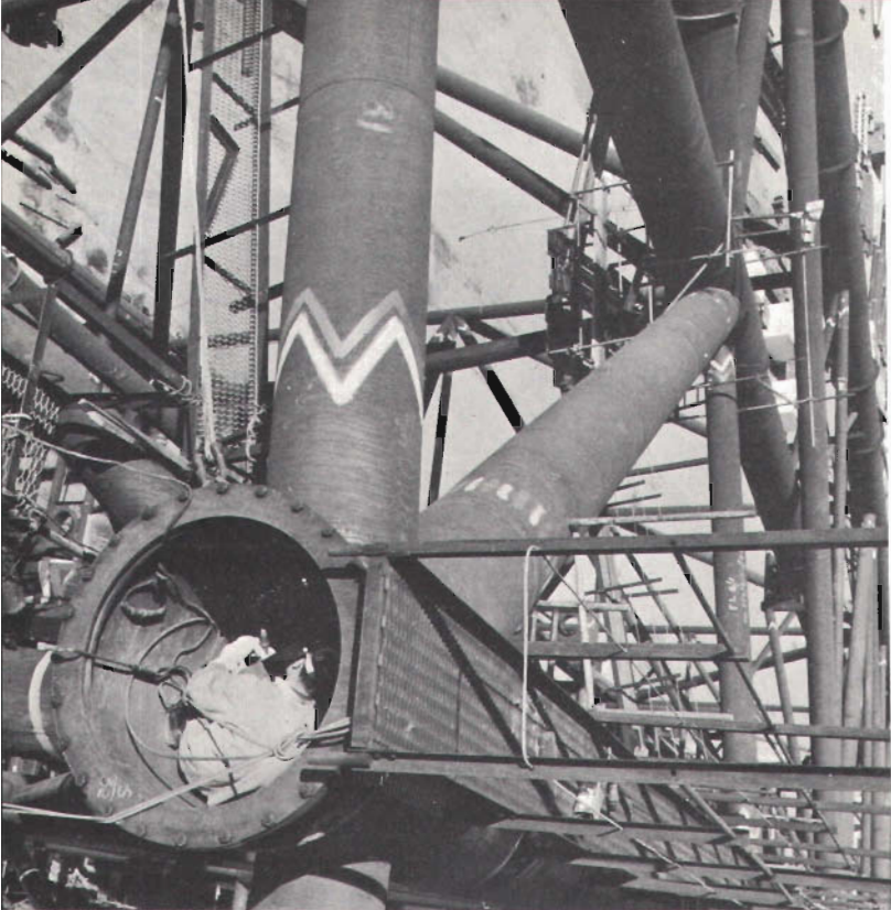
A welder at work inside one of the hollow steel legs of the Kingfish platform jacket during construction.
